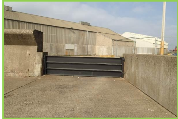
New flood boards at access point in crest wall. (Asset Ref. No. 121AB901B0802C04)
