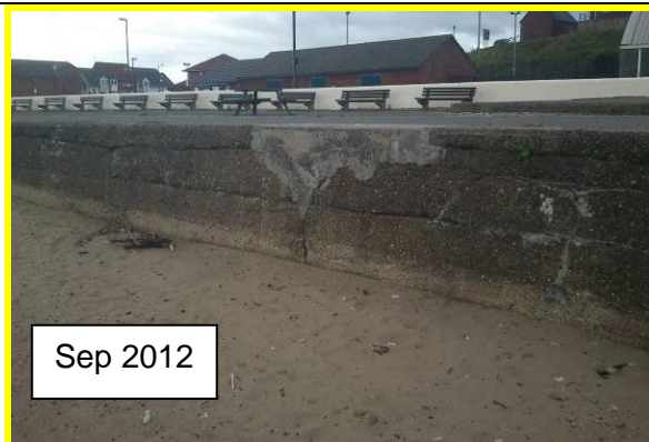
Multiple horizontal cracks and previous repairs in concrete wall. (Asset Ref. No. 121AB901B0702C01)
