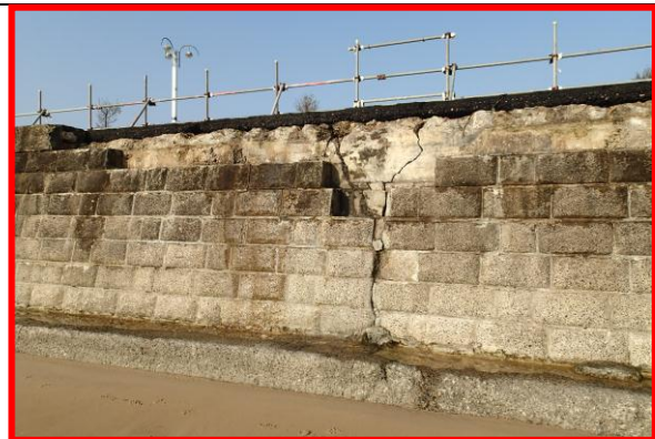
Storm damage to seawall at Seaburn. (Asset Ref. No. 121AB901B0603C02)
