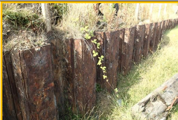
Badly corroded sheet pile defence at south west side of former South Outlet basin. (Asset Ref. No. 121AB901B0802C07)
