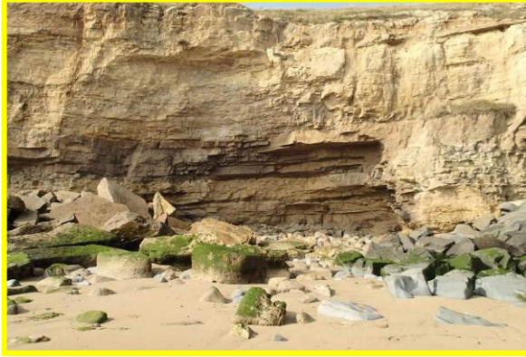
Caves forming in cliff toe at southern end rock armour to the south end of Hendon Seawall. (Asset Ref. No. 121AB901B0803C01)
