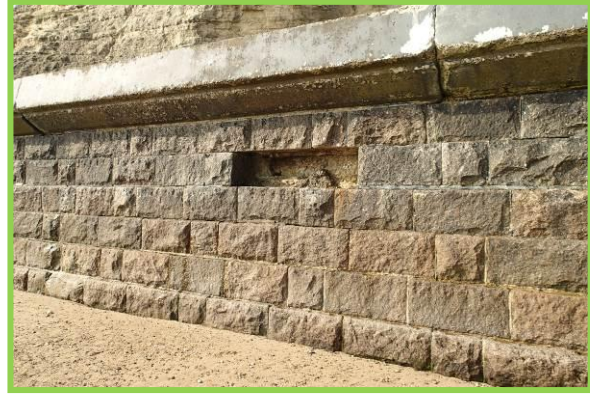
Missing block on most exposed seaward extent of the wall. (Asset Ref. No. 121AB901B0605C01)
