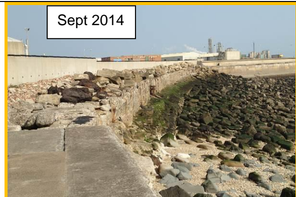
Defence rock armour in similar or slightly worse condition than in 2013. (Asset Ref. No. 121AB901B0802C03)
