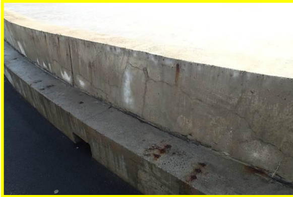
Crest wall cracks and rust staining at fixings from previous seats. (Asset Ref. No. 121AB901B0603C03)
