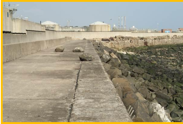
Small rock armour units washed onto crest slab causing storm damage. (Asset Ref. No. 121AB901B0802C02)
