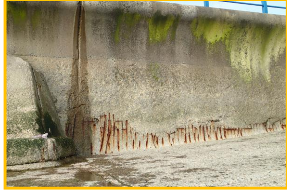
Abrasion of wall exposing reinforcement. (Asset Ref. No. 121AB901B0803C02)
