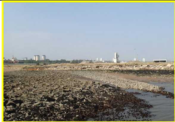
Random demolition rubble tipped into old dock (Asset Ref. No. 121AB901B0801C08)
