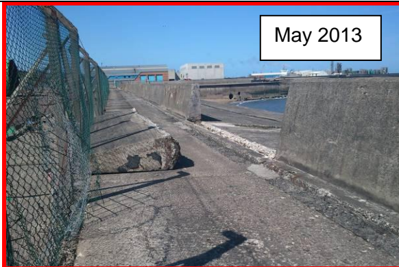
Failed section of crest wall. (Asset Ref. No. 121AB901B0802C01)
