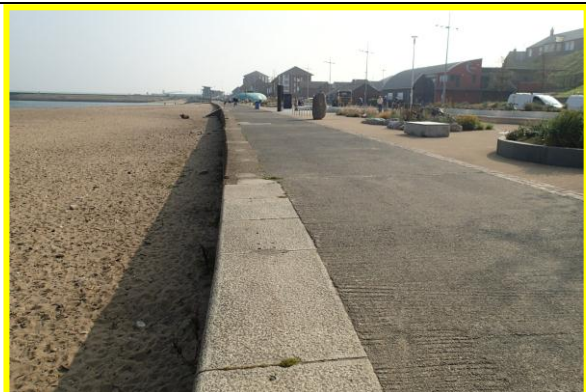
Roker beach promenade in fair condition. Area to rear has been resurfaced under regeneration scheme.
