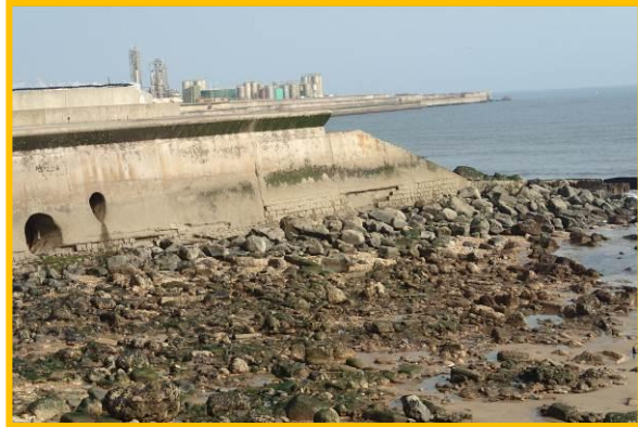
Missing facing masonry requires attention. (Asset Ref. No. 121AB901B0802C01)
