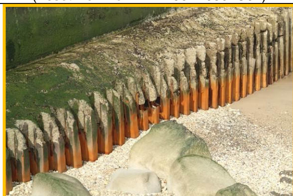
Badly abraded toe piles near south end of defence showing holes through to voids in wall. (Asset Ref. No. 121AB901B0802C01)
