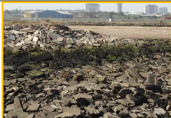
Random demolition rubble tipped into old dock to rear of South West breakwater. (Asset Ref. No. 121AB901B0802C06)
