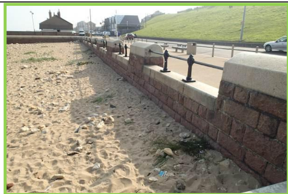
Southern section of wall protected by wide beach in good overall condition. (Asset Ref. No. 121AB901B0605C02)
