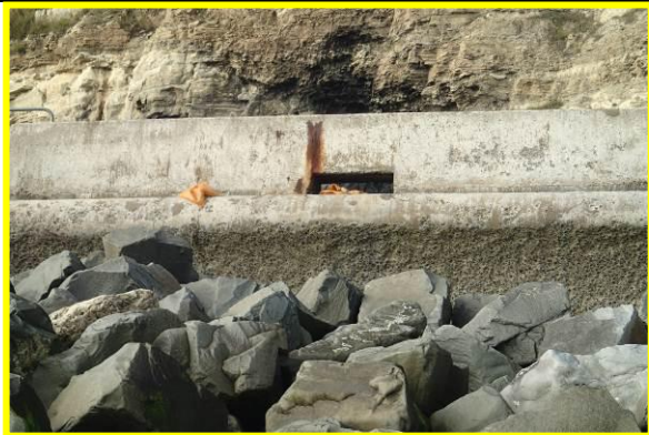
Crest wall with corrosion around enlarged drainage holes towards southern end of defence. (Asset Ref. No. 121AB901B0803C02)
