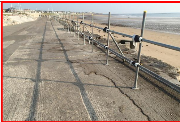
Storm damage to promenade. (Asset Ref. No. 121AB901B0603C02)
