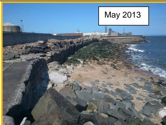
Loosely stacked rock armour on crest and at toe provides limited protection. (Asset Ref. No. 121AB901B0802C03)
