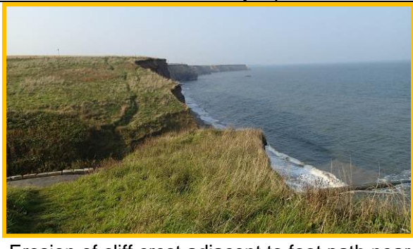
Erosion of cliff crest adjacent to foot path near Ryhope dene (Asset Ref. No. 121AB901B0804C02)
