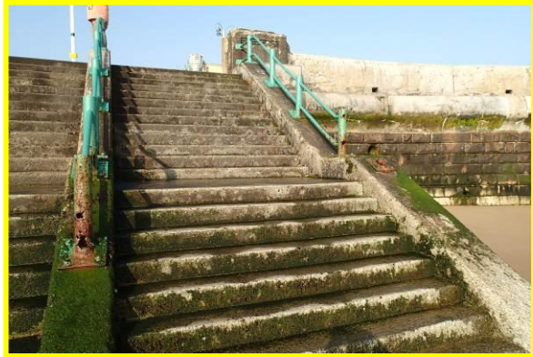
Heavily corroded hand rails to south steps at traffic roundabout, with seaward section missing. (Asset Ref. No. 121AB901B0603C03/C02)
