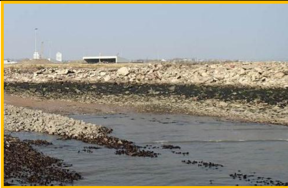
Tipped rubble at landward end of North East Pier protecting inner face of defence. (Asset Ref. No. 121AB901B0801C07)
