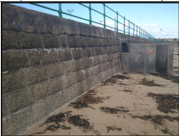
Photo from 2012 report. (Asset Ref. No. 121AB901B0603C02)
