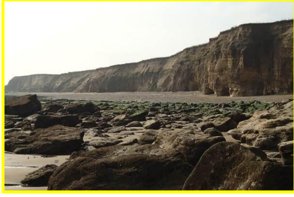
Cliffs south of Hendon are afforded a degree of natural protection by rubble and small beach at toe. (Asset Ref. No. 121AB901B0803C01)
