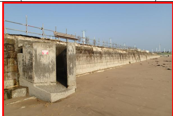
Failed coping adjacent to northern outfall. (Asset Ref. No. 121AB901B0603C02)
