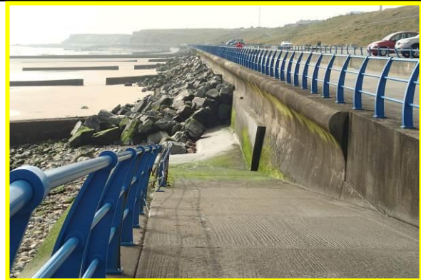
Wall and handrails and rock armour in good condition but defence has badly corroded toe piles; northern section of defence. (Asset Ref. No. 121AB901B0803C02)
