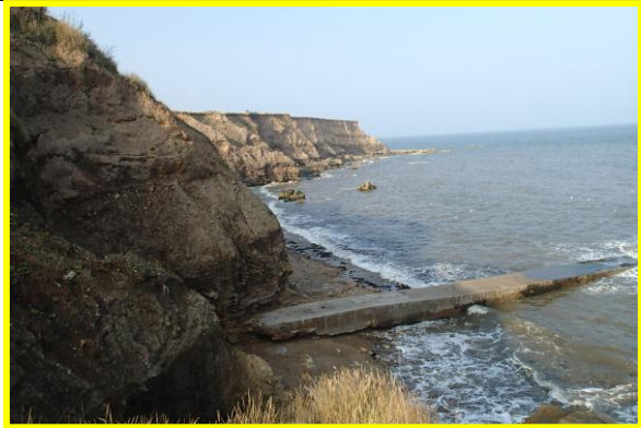
Mud slides and active erosion in upper till cliff. Also shows undermined concrete cladding on outfall structure at Ryhope Nook. (Asset Ref. No. 121AB901B0804C03)
