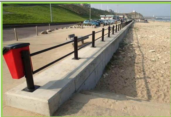
Low concrete encased wall at Marine Walk in good overall condition. (Asset Ref. No. 121AB901B0605C02)
