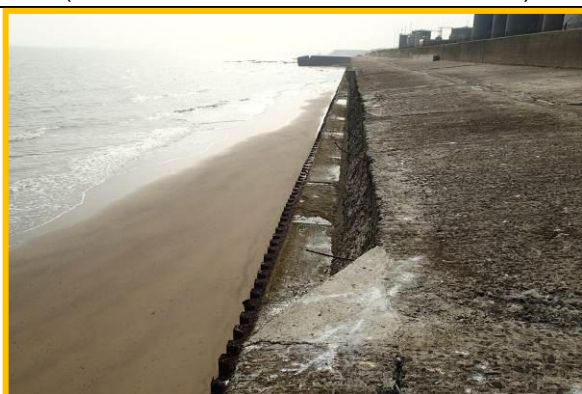
Missing section of coping at seaward edge of crest slab. (Asset Ref. No. 121AB901B0802C01)
