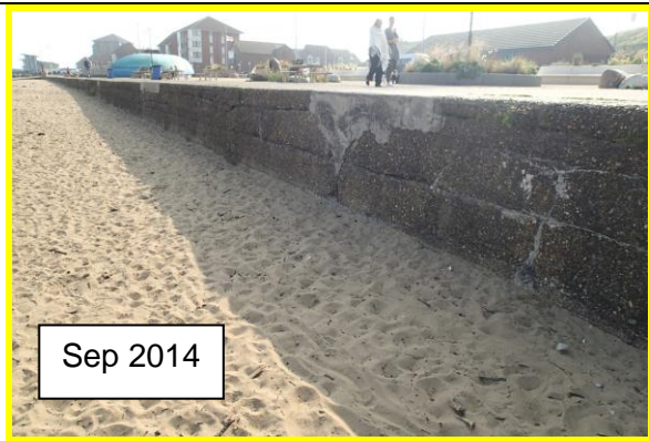
No change to cracks in wall, but beach level slightly higher. (Asset Ref. No. 121AB901B0702C01)
